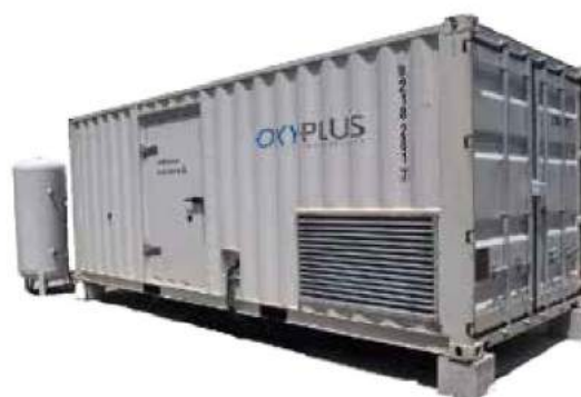
In container equipped with power cabinet, ventilation and lighting
